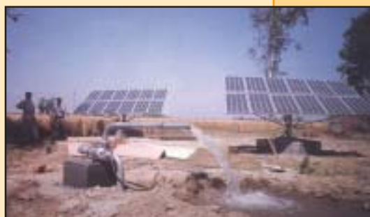
Solar PV water pumping system
